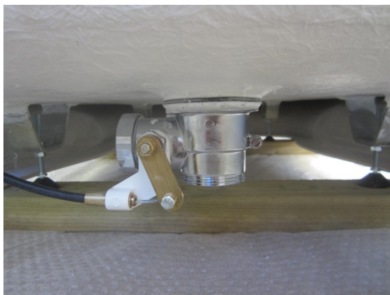
Bespoke waste assembly beneath the pool.
